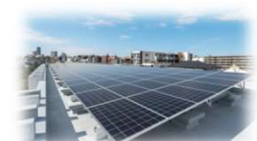
Mega solar power plants
